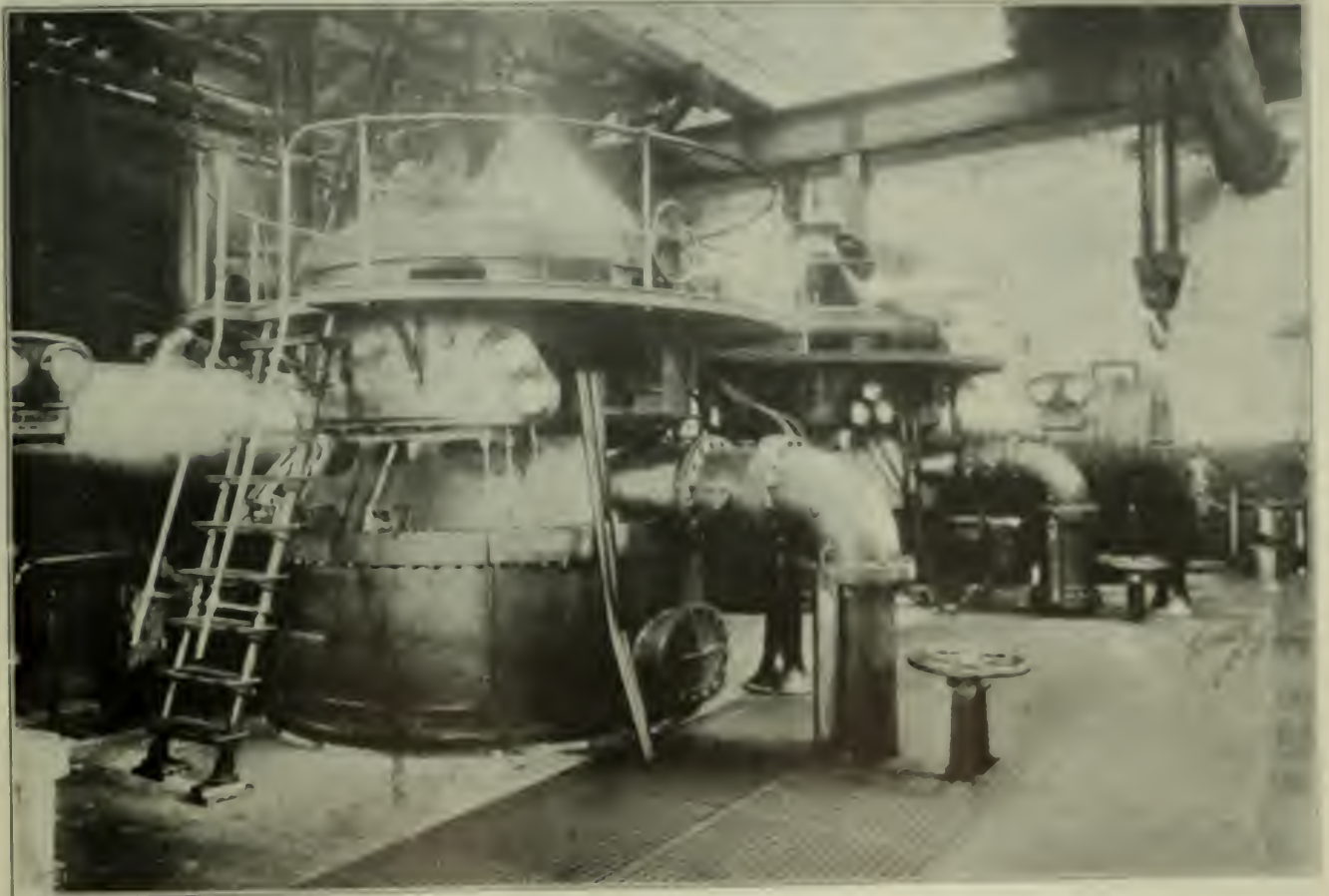
FIG. 1. LIVE-PRESSURE SEA-KILN-WAY TURBINE INSTALLATION IN PHILADELPHIA RAILWAY POWER HOUSE.
